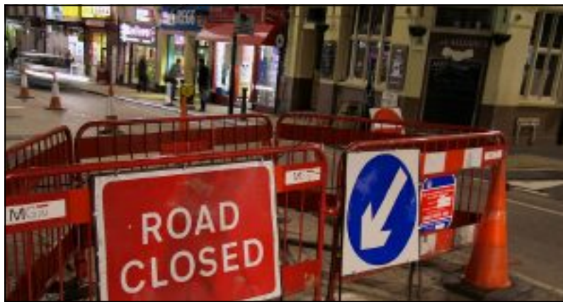
TRAFFIC NIGHTMARE: Roadworks are set to continue at the junction of Selhurst Road and Oliver Grove in South Norwood while Victorian water mains are replaced Photo no: CRCDC201201198
