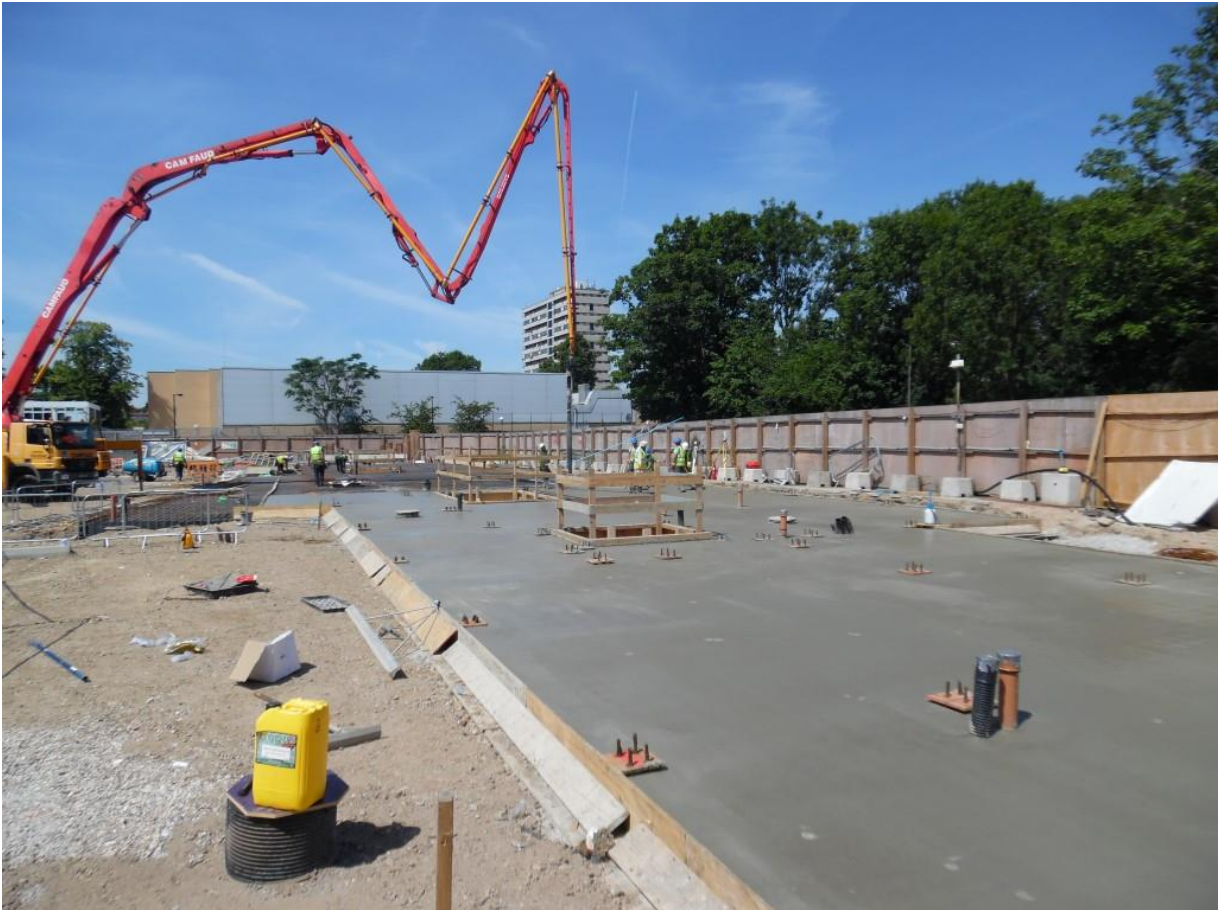
Image 05, 07-07-2017; pumping concrete to ground floor in the background, completed slab in foreground
