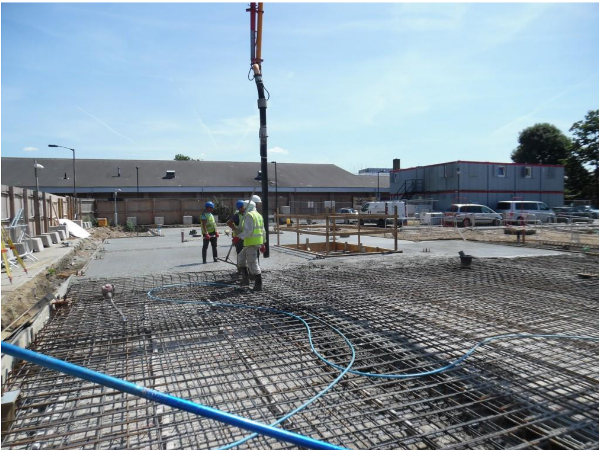
Image 02, 07-07-2017; discharging concrete via pump to large expanse of the structural ground floor slab
