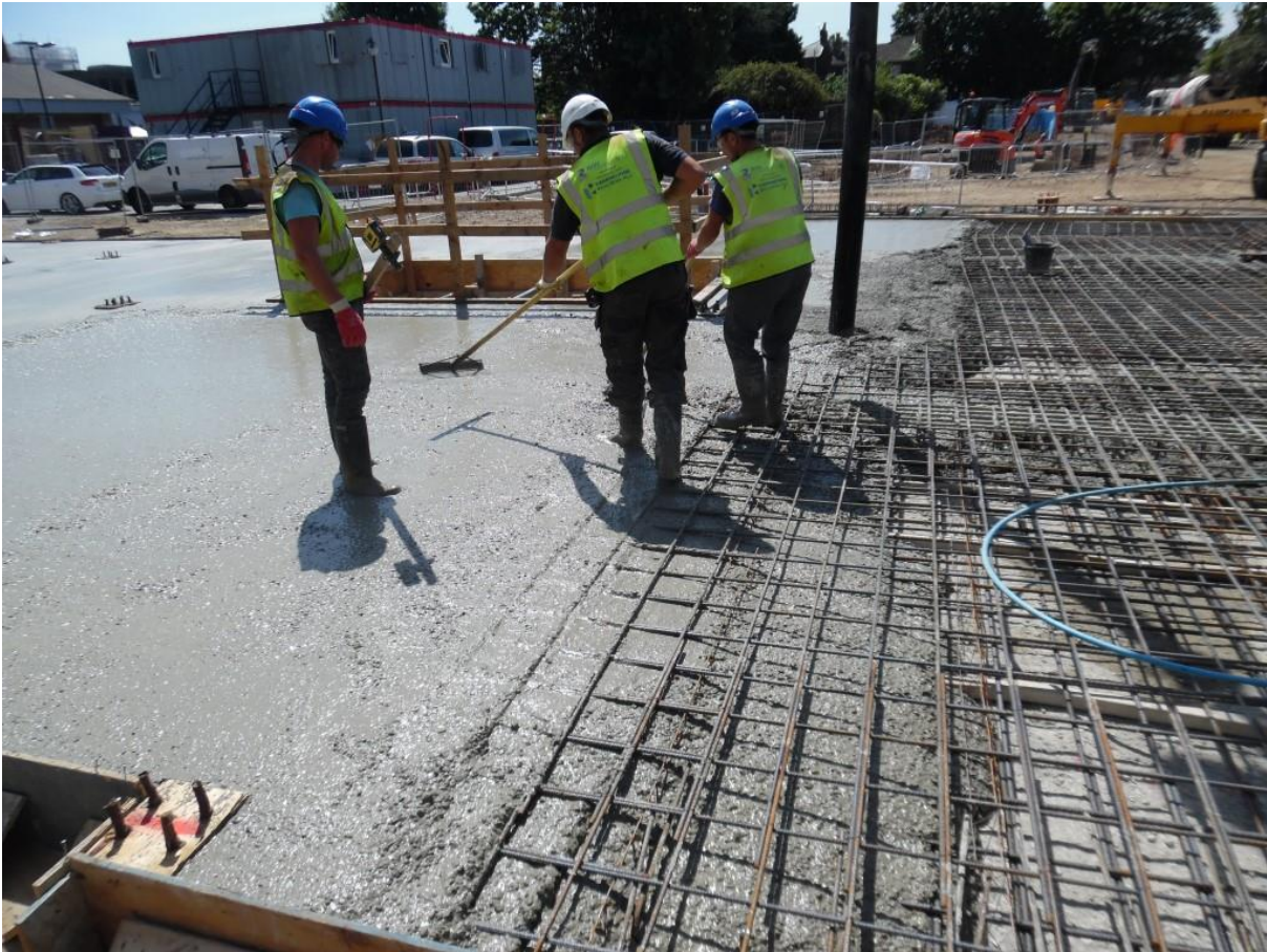
Image 03, 07-07-2017; distributing the wet concrete mix into position, vibrating concrete as work proceeds
