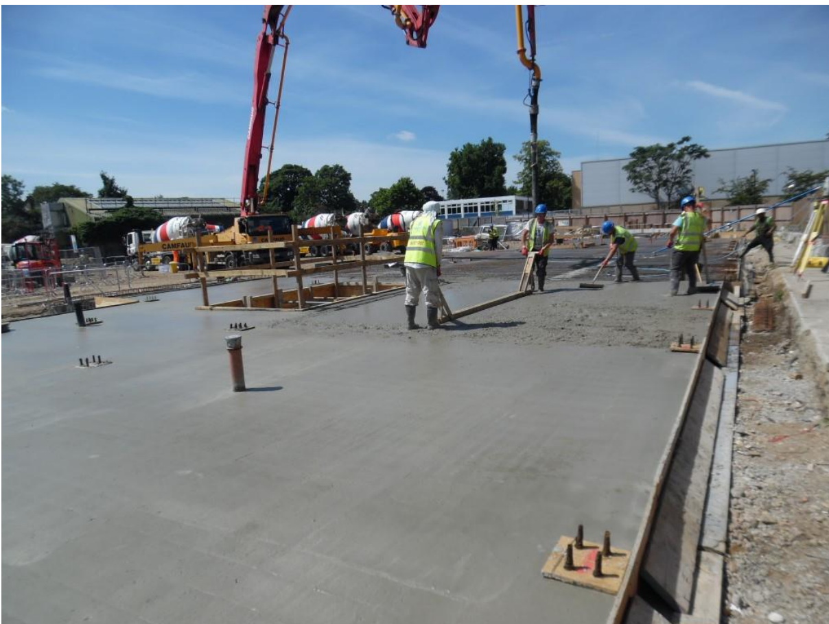
Image 0, 07-07-2017; tamping & levelling the concrete using screed method, laser level employed for flatness
