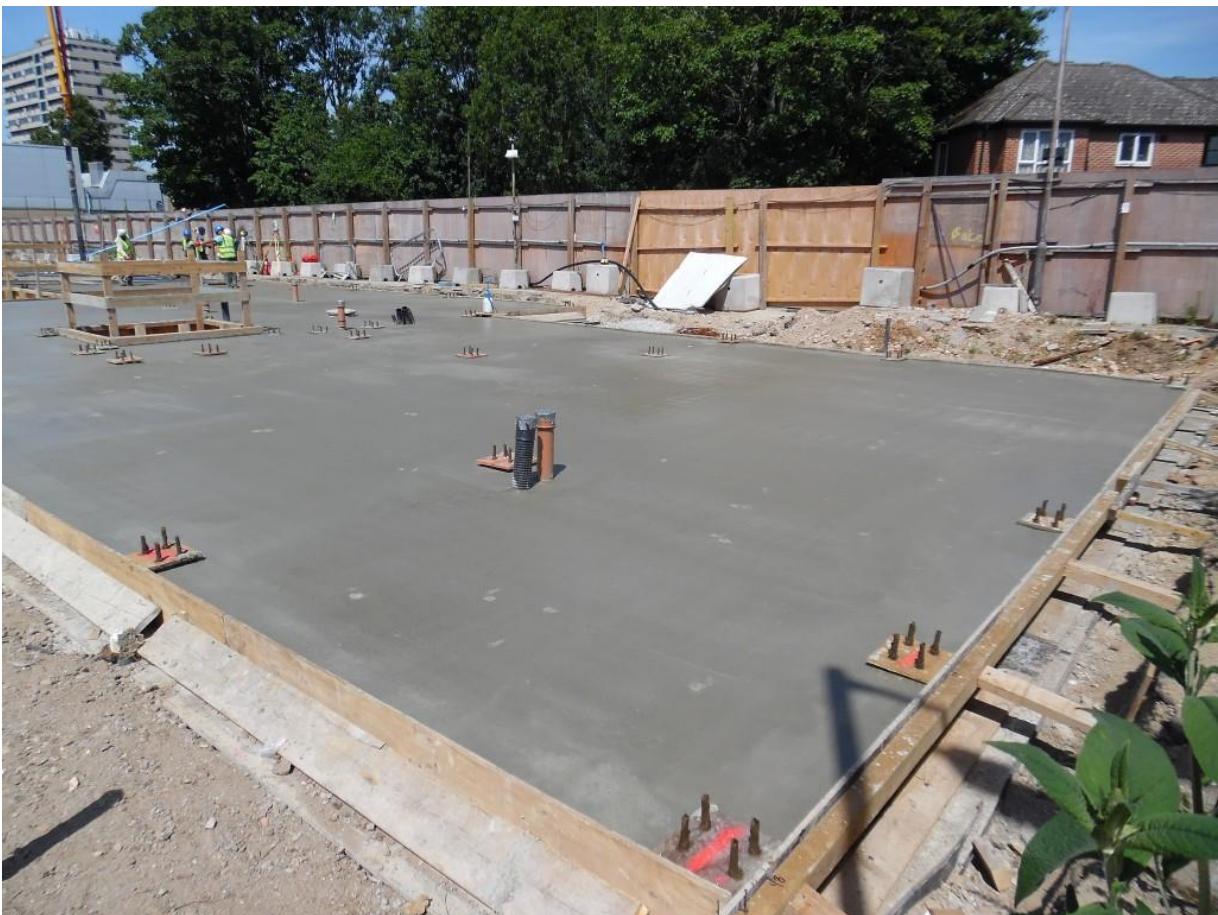
Image 06, 07-07-2017; concrete slab trowelled off flat to north-east corner of building, spray cure to surface
